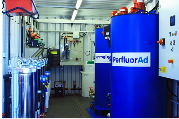
Figure 8. Mobile PerfluorAd system - built into 20 'containers - for temporary use for the treatment of PFAS contaminated water
