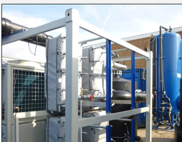
Vapour Conditioning System
