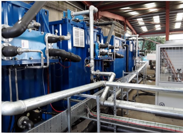
MPE System + Heat Exchangers
