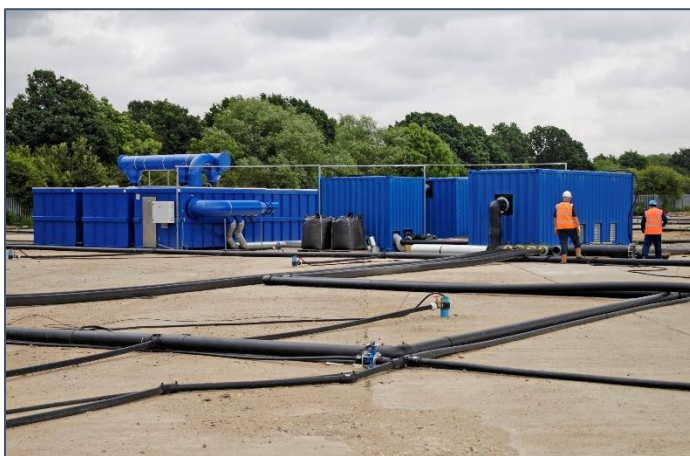
5000m 3 /hr SVE system with Biofilter and 75 Pneumatic Total Fluids Pumps
