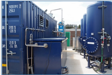
Pump & Treat System
